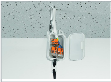
Pendant light connection in a suspended ceiling
