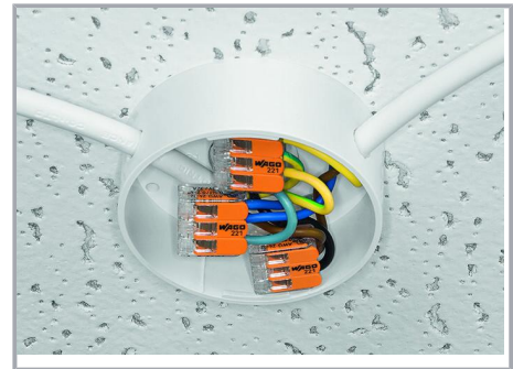
Lighting distribution in a ceiling canopy
